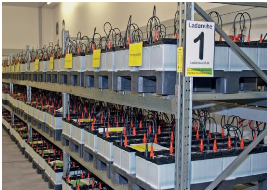
Battery Care Station Seesen Ladereihe / Foto: akkuteam
